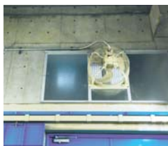
Forced ventilation fan
