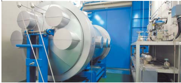
Explosion-resistant chamber/ Pressure and flow control unit
