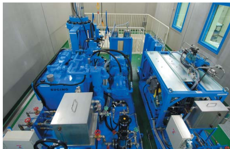
Hydraulic pressure test equipment
